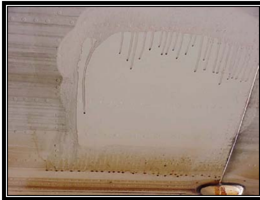
Figure 1: Note beading of dirt on previously cleaned surface.
